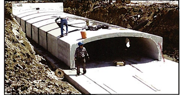
6 Joint Seal – Commercial joint wrap is applied as a seal between precast units.
