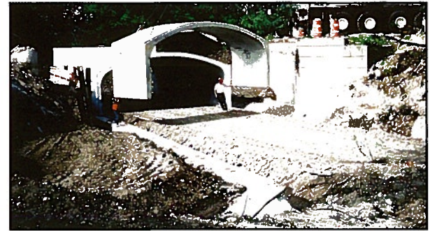
5 Foundation – Strip footings or slab base can be either cast in place or precast.
